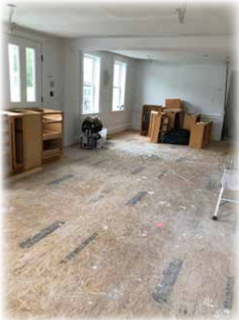
The third phase renovation (in progress) will create a large public gathering space while improving the building's flow and functionality.
